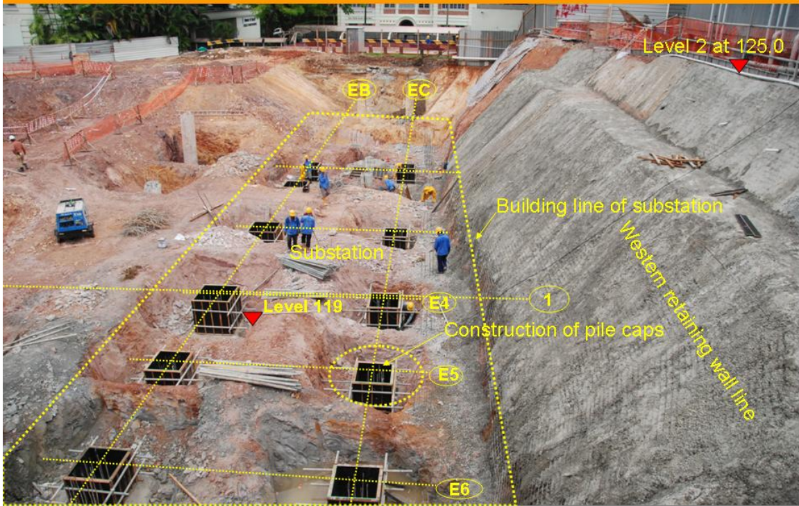
25 June 2007 - PUB Substation at the South-West corner
