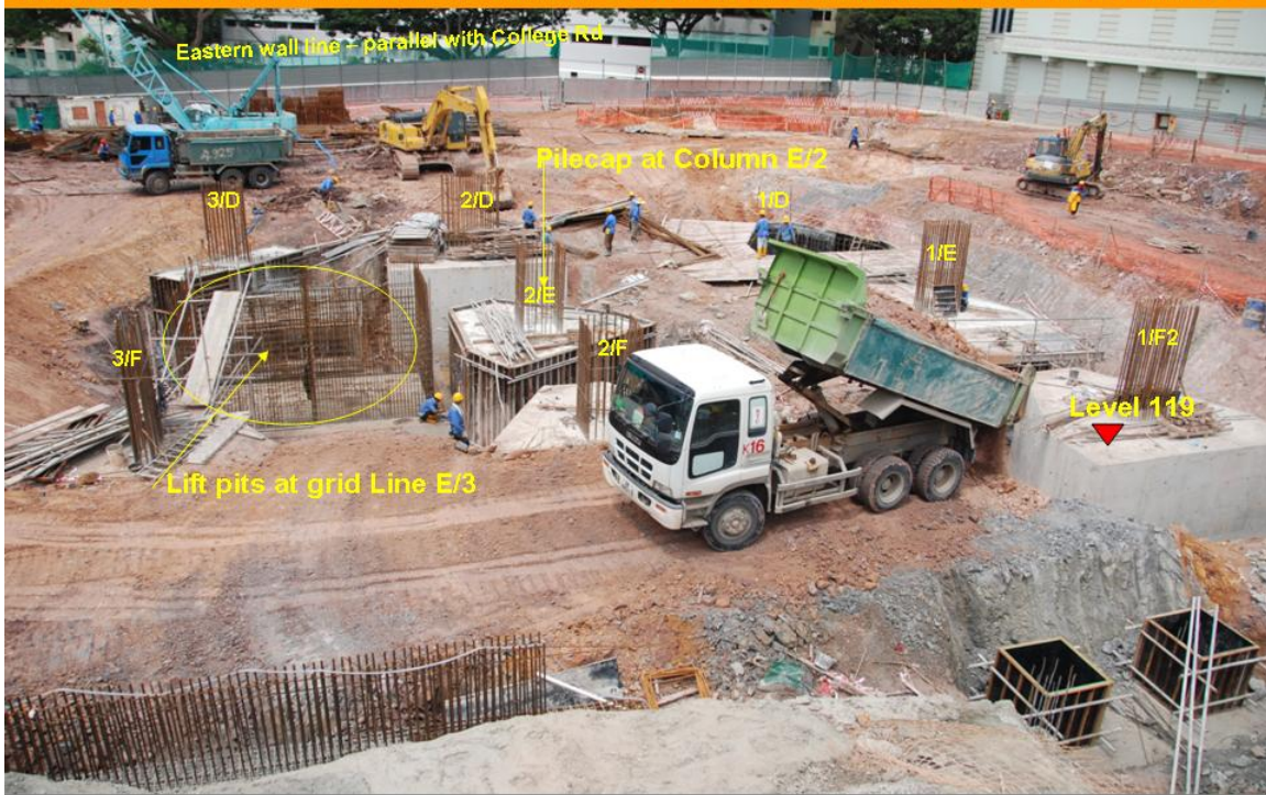
Pile caps at grid F/1,2&3, E/1,2&3 and D/2&3 are completed. D/1 is still in progress.
